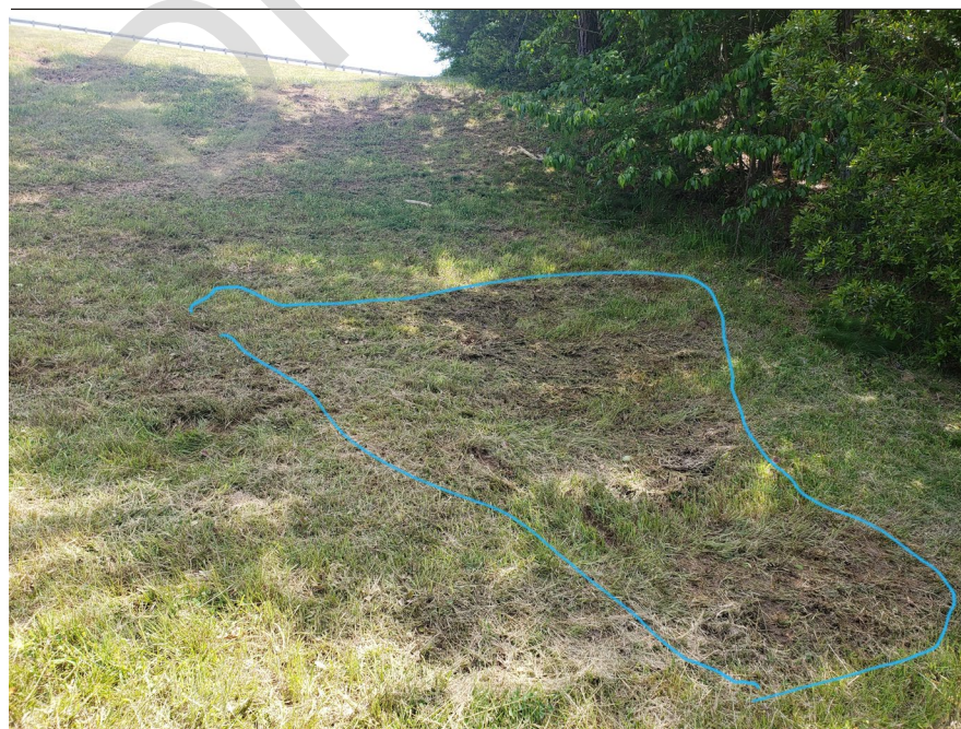
Photograph 4: Left Abutment, May 2020 – wet spot observed on the left side of the abutment (from approximately STA 1+95 to 2+05).
