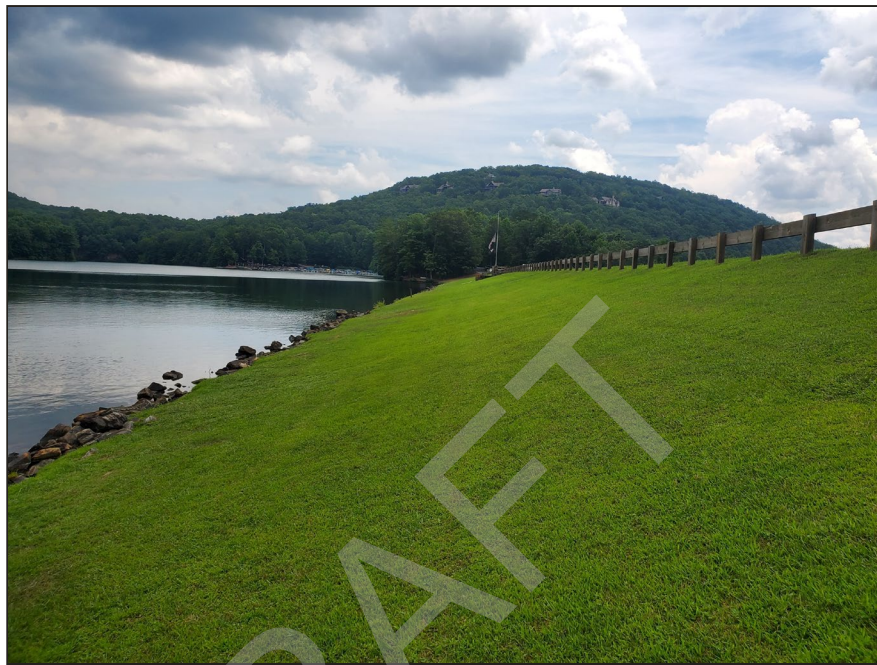
Photograph 1: Upstream Face, July 2020 – localized areas of erosion and beaching along shoreline.
