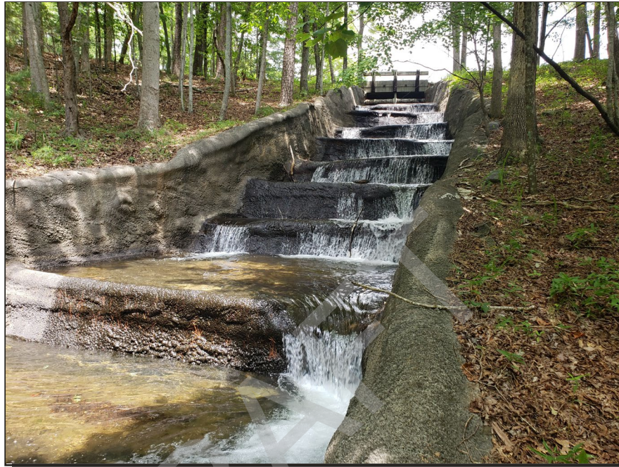
Photograph 3: Spillway, July 2020 – general view of stepped spillway with moderate flow, and tree limbs and debris noted during inspection.
