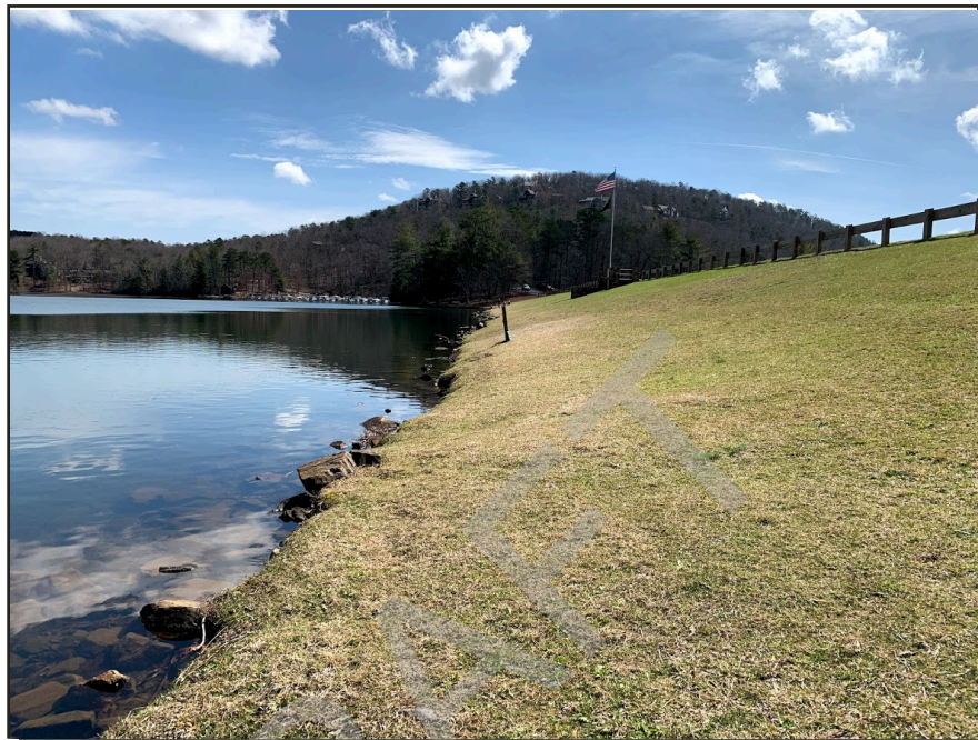
Photograph 1: Upstream Face, May 2020 – localized areas of erosion and beaching along shoreline.
