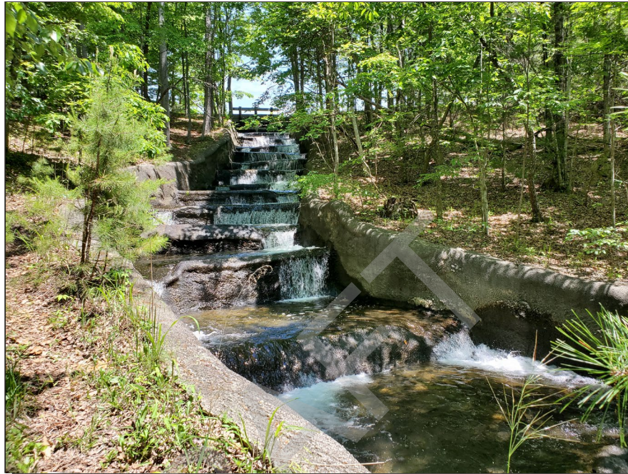
Photograph 3: Spillway, May 2020 – general view of stepped spillway with moderate flow, and tree limbs and debris noted during inspection.
