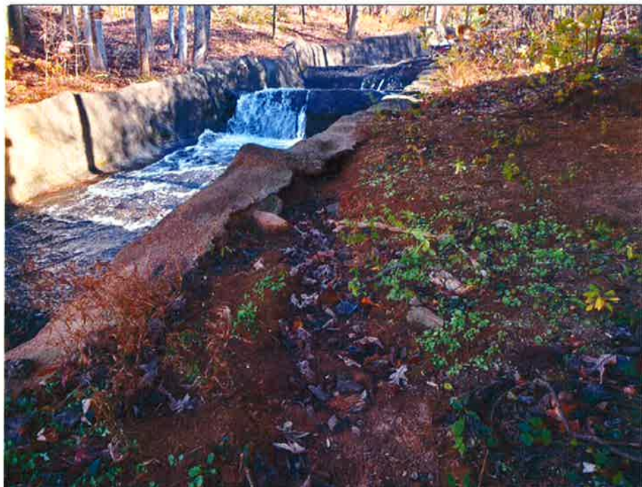
Photograph 4: Spillway, Nov. 2020 – Area of previously identified water flow behind concrete lined channel. Water flow was observed to continue but did not daylight at surface in depicted location.
