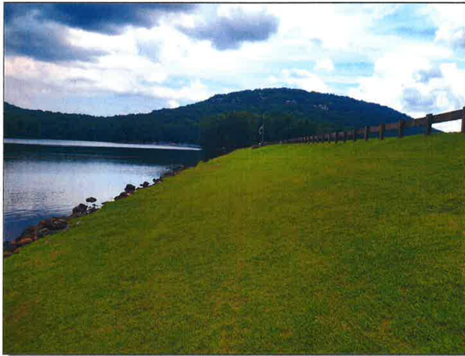
Photograph 1: Upstream Face, July 2020 – localized areas of erosion and beaching along shoreline.
