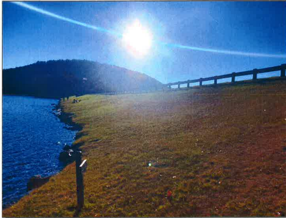
Photograph 1: Upstream Face, Nov. 2020 – localized areas of erosion and beaching along shoreline.
