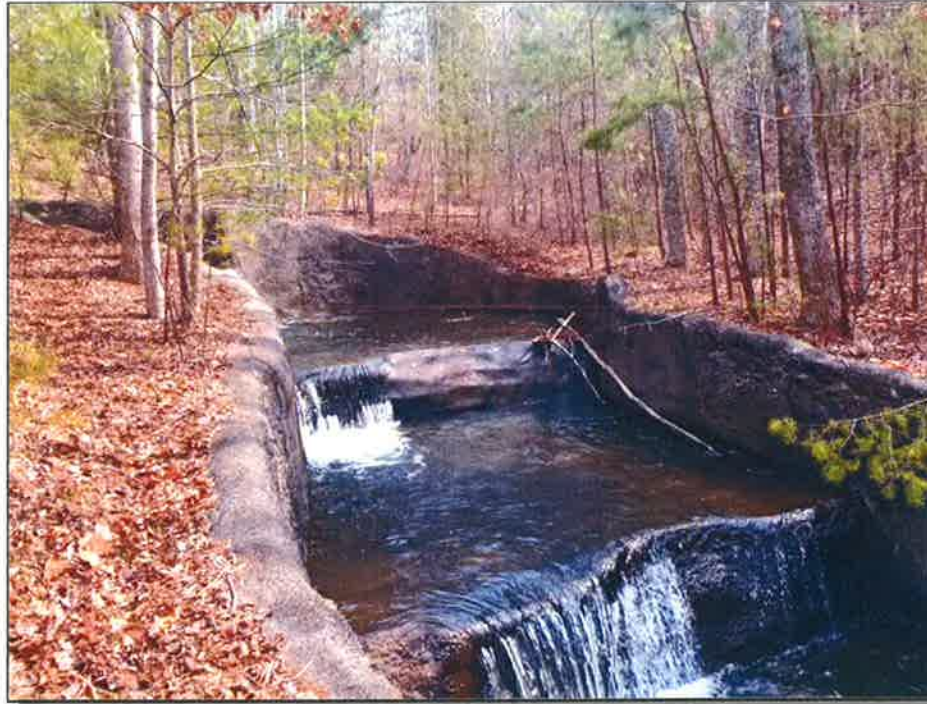
Photograph 3: Spillway, Mar. 2021 – general view of stepped spillway with moderate flow, and tree limbs and debris noted during inspection.
