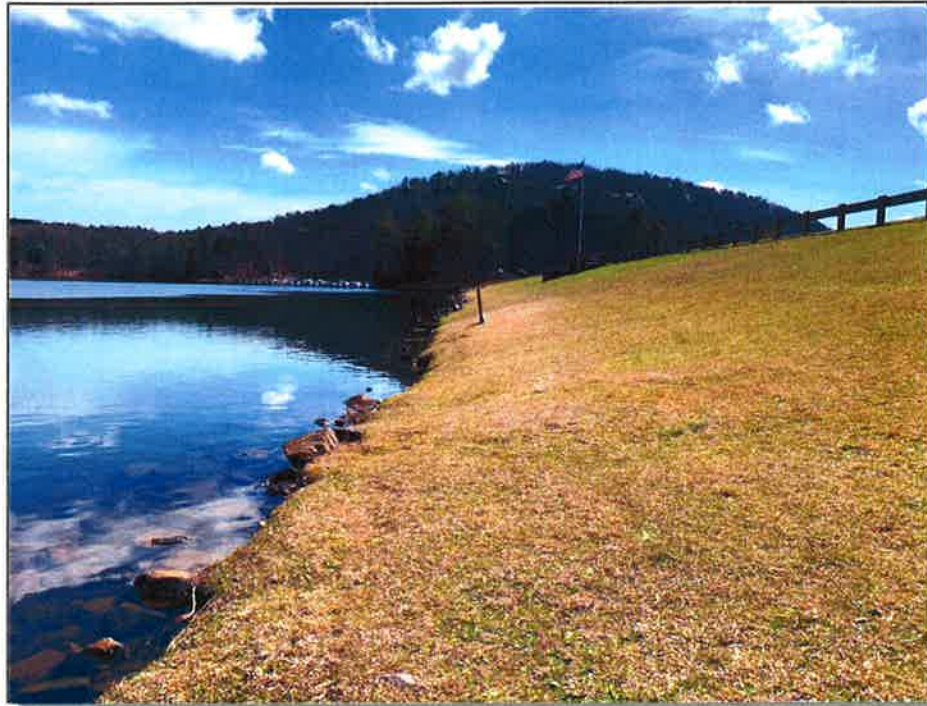
Photograph 1: Upstream Face, May 2020 – localized areas of erosion and beaching along shoreline.
