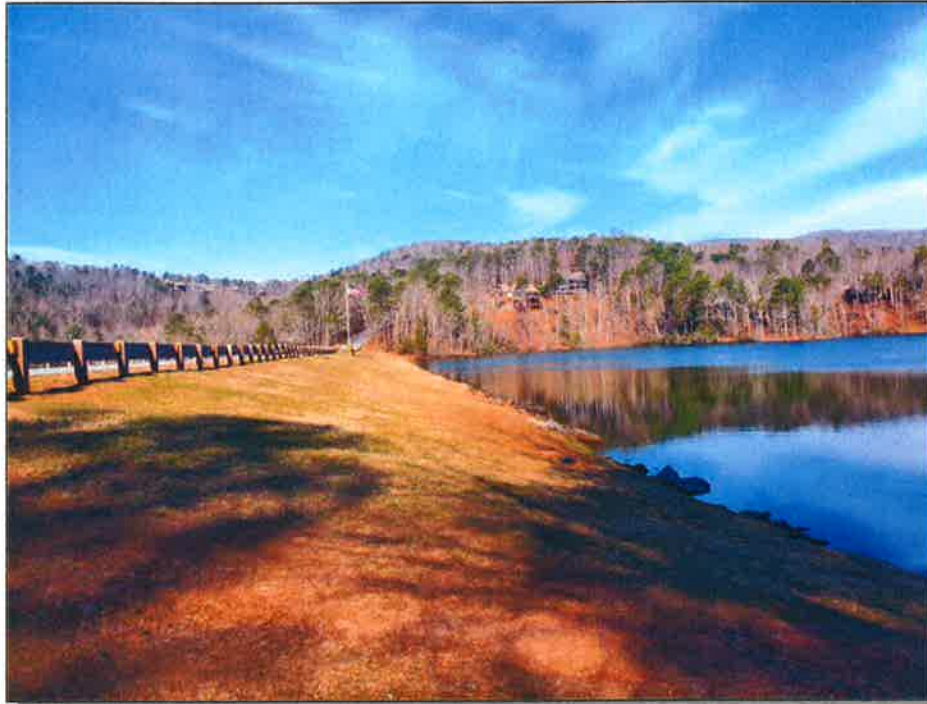
Photograph 1: Upstream Face, Mar. 2021 – localized areas of erosion and beaching along shoreline.
