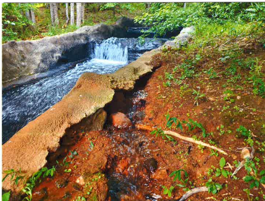
Photograph 4: Spillway, July 2020 – water flow observed behind the concrete lined channel.
