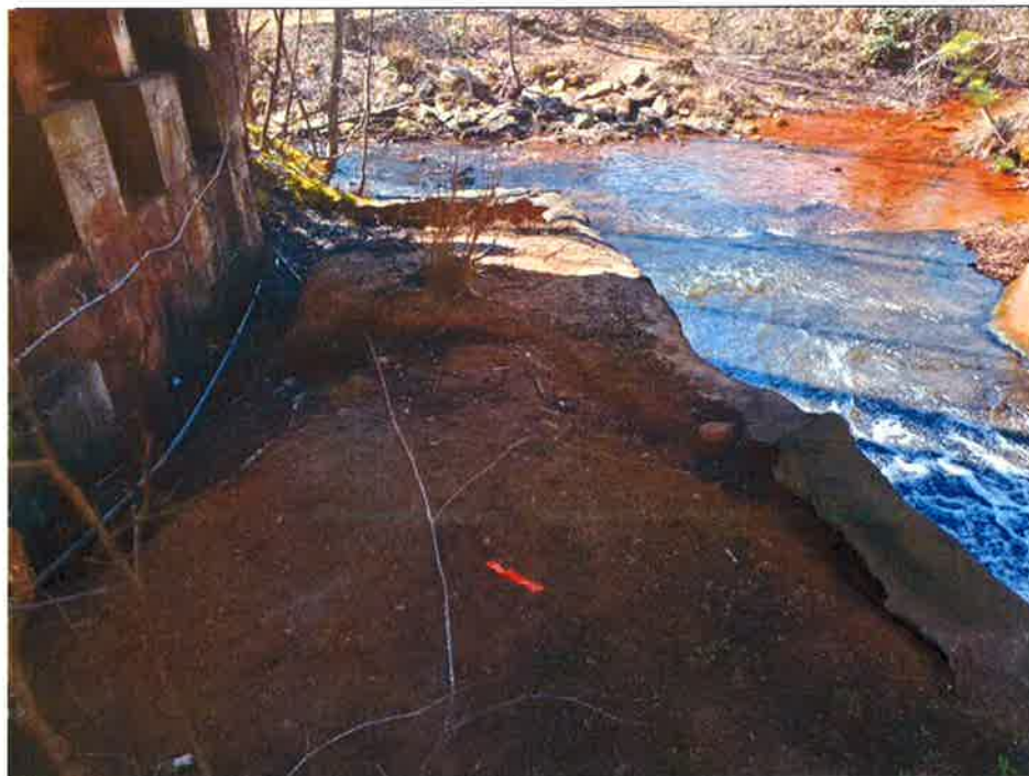
Photograph 4: Spillway, Mar. 2021 – area of previously identified water flow behind concrete lined channel. Water flow was observed to continue but did not daylight at surface in depicted location.
