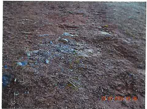
bare area on upstream slope
