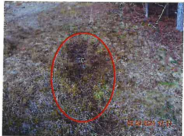
seepage on lower left abutment
