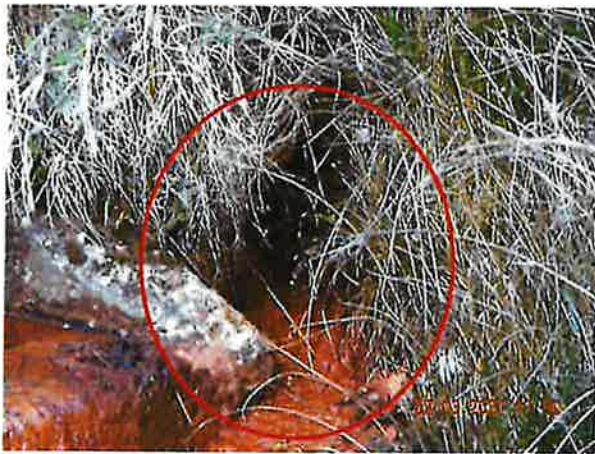
seepage from voidspace behind left wall at low-level outfall
