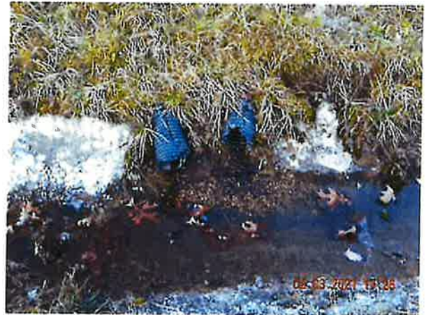
deteriorated black corrugated pipes draining into lower ditch
