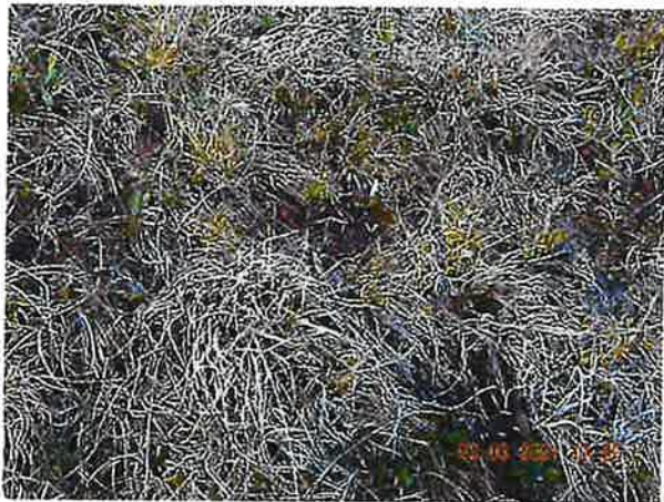
apparent seepage and soft ground on lower downstream slope
