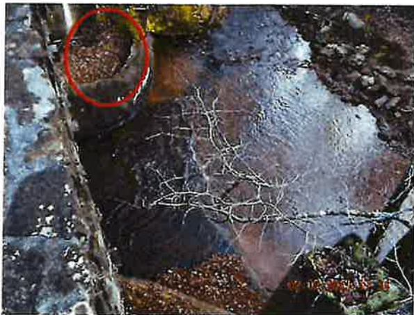
principal spillway plunge pool; notice voidspace behind left wall
