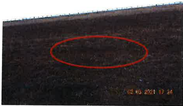
bare spots on lower downstream slope
