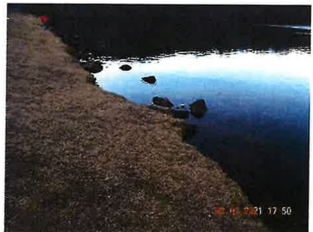
riprap displaced down upstream slope; wave-action erosion apparent
