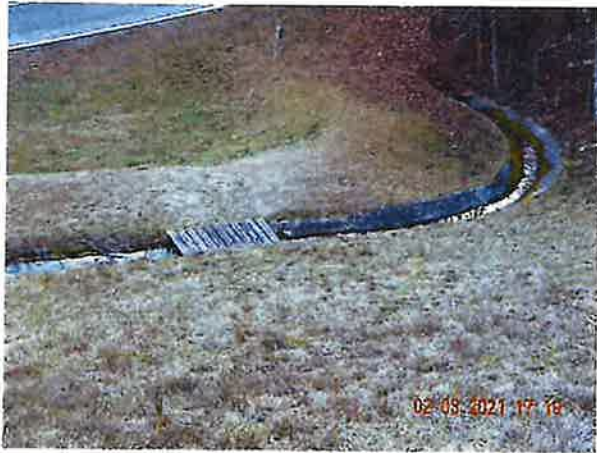
seepage flowing in ditch in lower downstream slope
