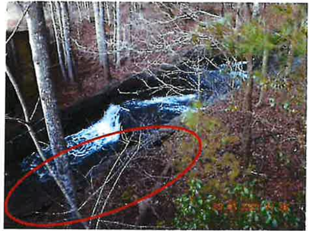
voidspace behind left wall along principal spillway
