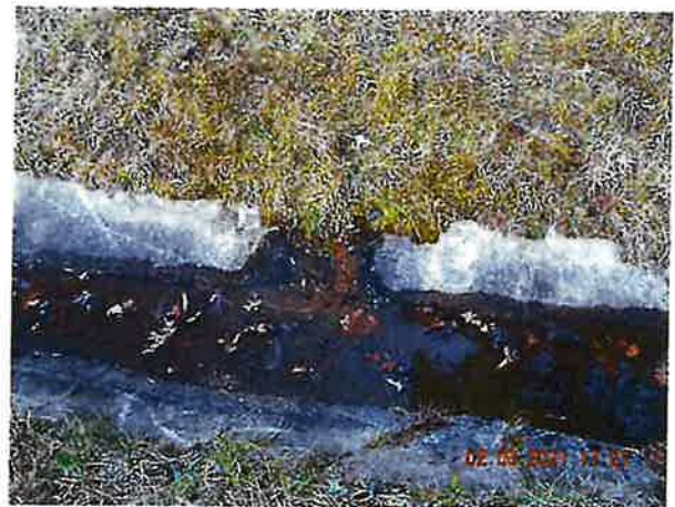
seepage into lower ditch
