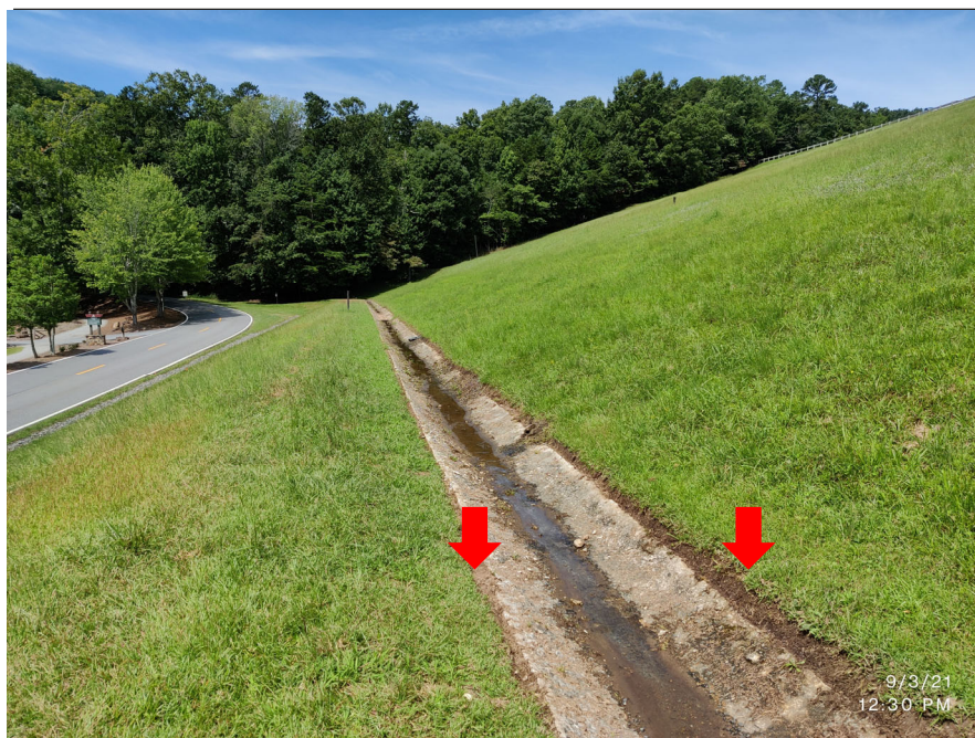
Photograph 8: Edging performed on the concrete channels located on Bench No.1 and Bench No.2
