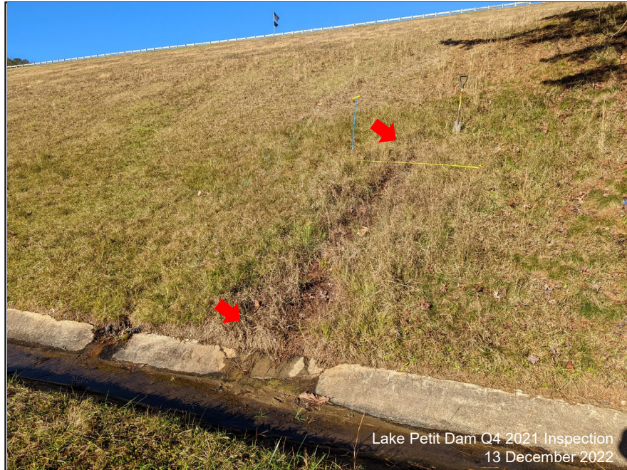
Photograph 5: Downstream Face, Dec. 2021 – Previously identified wet area above Bench No. 1. No changes observed in the wet spot.
