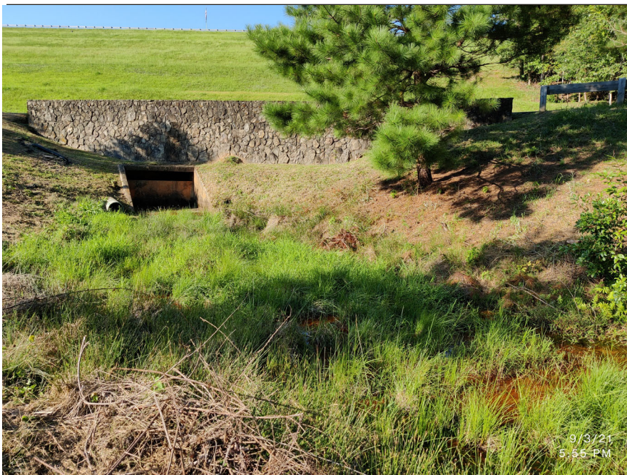
Photograph 6: Concrete distilling basin, Sept. 2021 – Vegetation clearing was conducted along the left and right banks.
