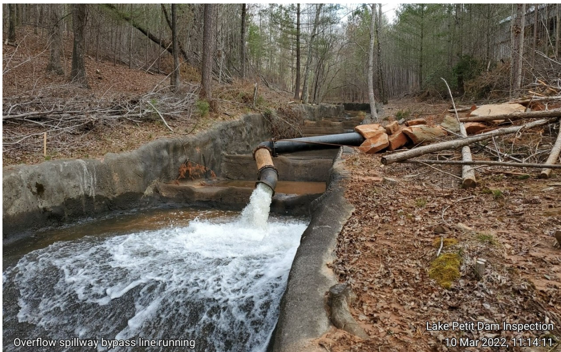
Photograph 28: Spillway bypass line in operation to lower reservoir level for maintenance repairs
