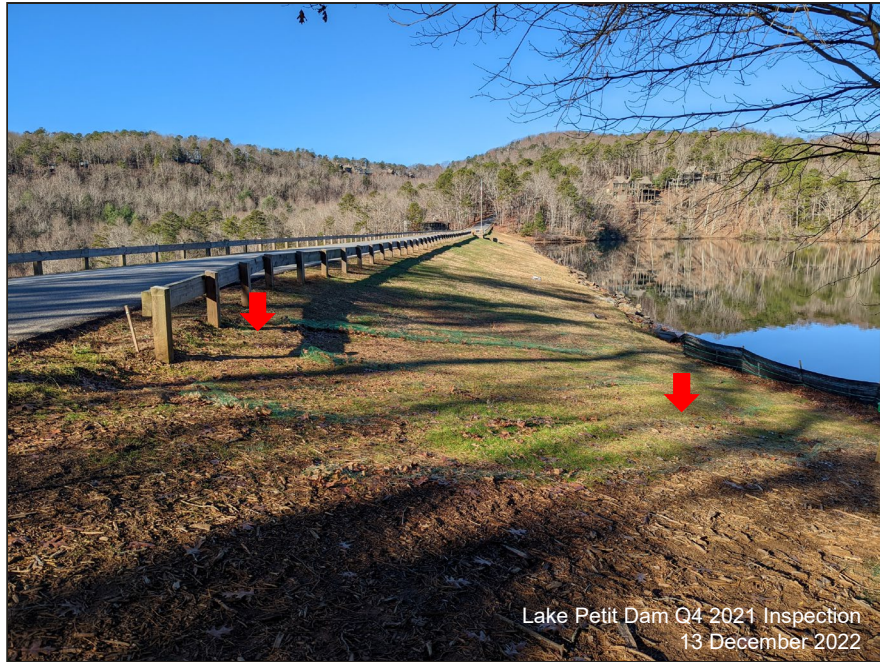
Photograph 1: Upstream Face, Dec. 2021 – Localized areas of surficial erosion previously repaired which require upkeep due to pedestrian traffic.
