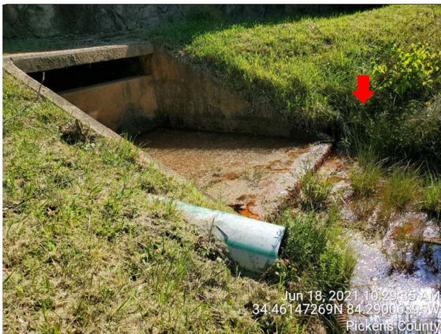
Photograph 8: Downstream outlet structure, Jun. 2021 – Normal flow observed exiting drainpipes from the impact-style stilling basin. Clear flow observed from a drainpipe at the lower right of photo (not visible). Other pipes adjacent to and downstream could not be observed due to overgrown vegetation.
