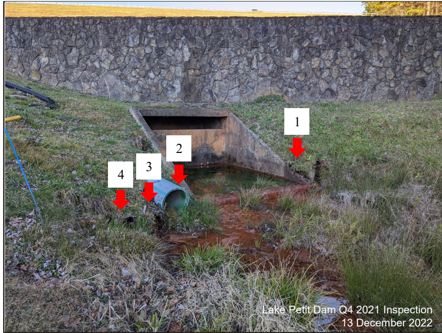
Photograph 7: Concrete Stilling Basin, Dec. 2021 – Flow observed and measured at the drain left of the concrete stilling basin (1), and the two corrugated pipes on the right (3 and 4).
