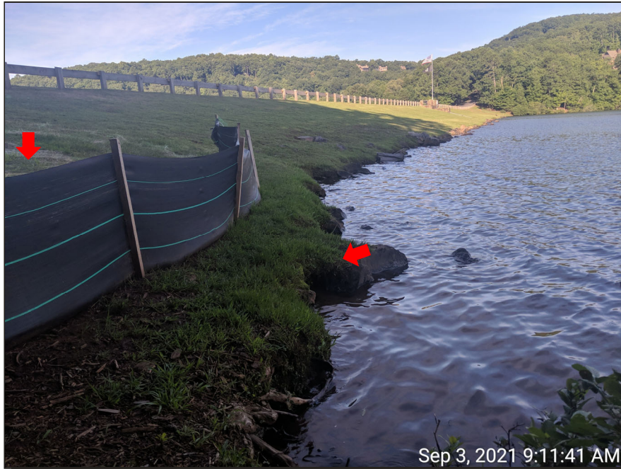
Photograph 1: Upstream Face, Sept. 2021 – localized areas of erosion repaired; beaching observed along shoreline.
