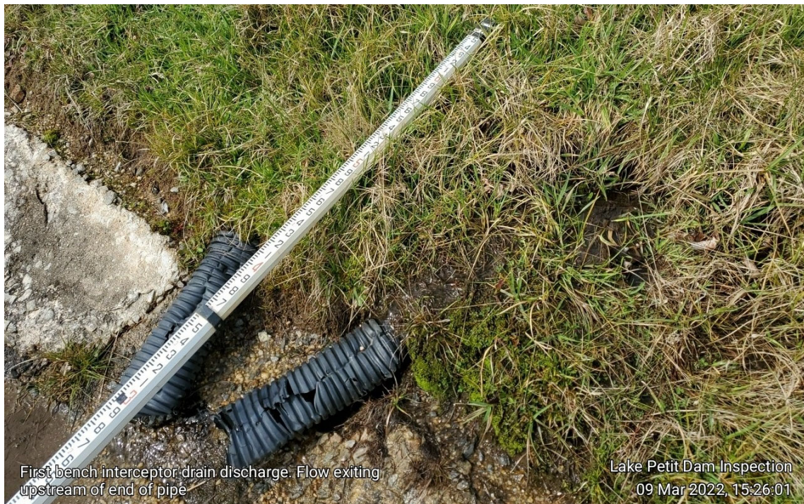
Photograph 17: Interceptor drains 9 and 10 discharge above end of pipe
