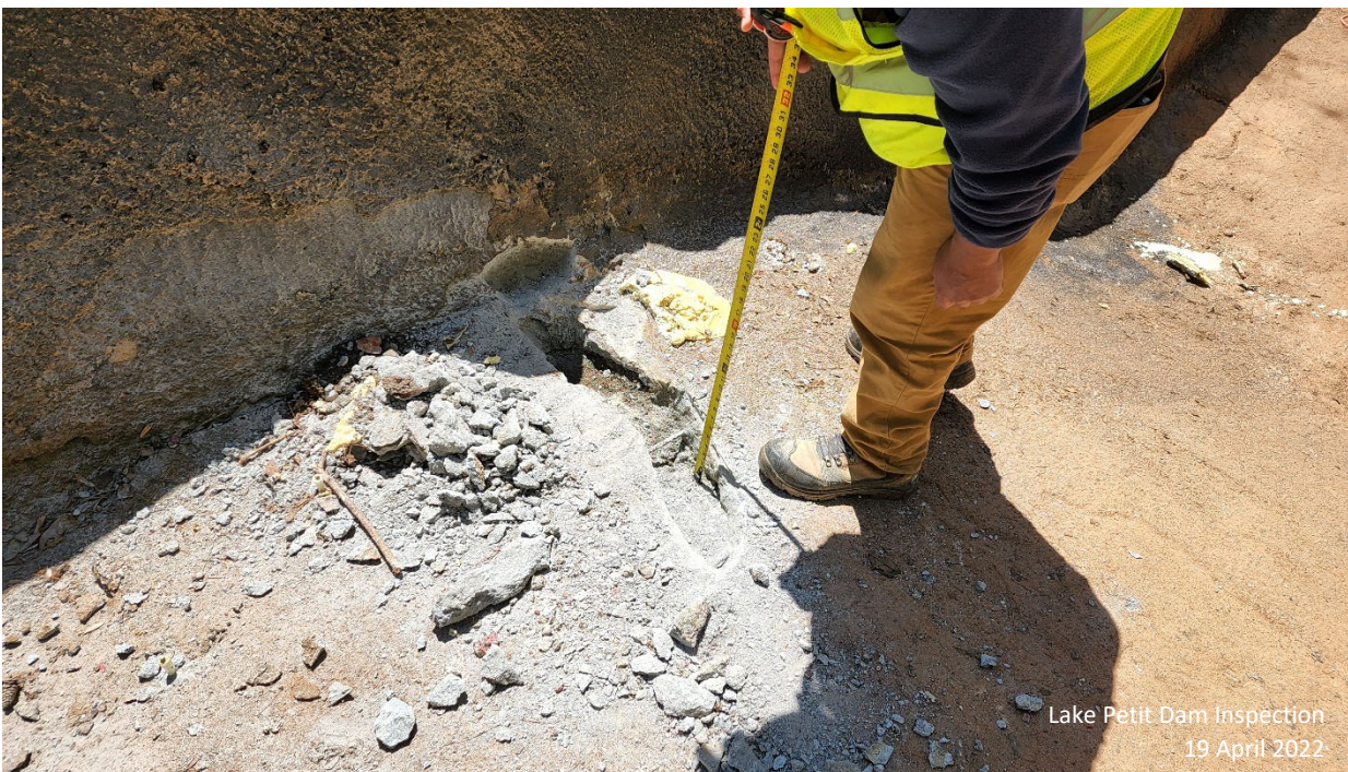
Photograph 34: Cracked area chipped out for patching
