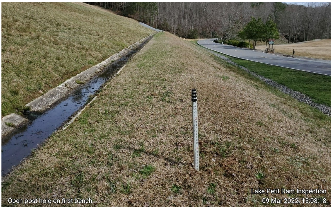
Photograph 13: Signpost hole in Bench 1 (El. 1544)
