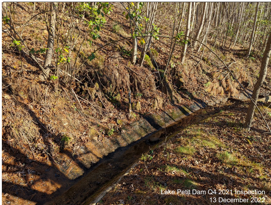
Photograph 6: Downstream Face, Dec. 2021 – Surficial erosion observed on the left abutment, which leads to sediment built in the left weir.
