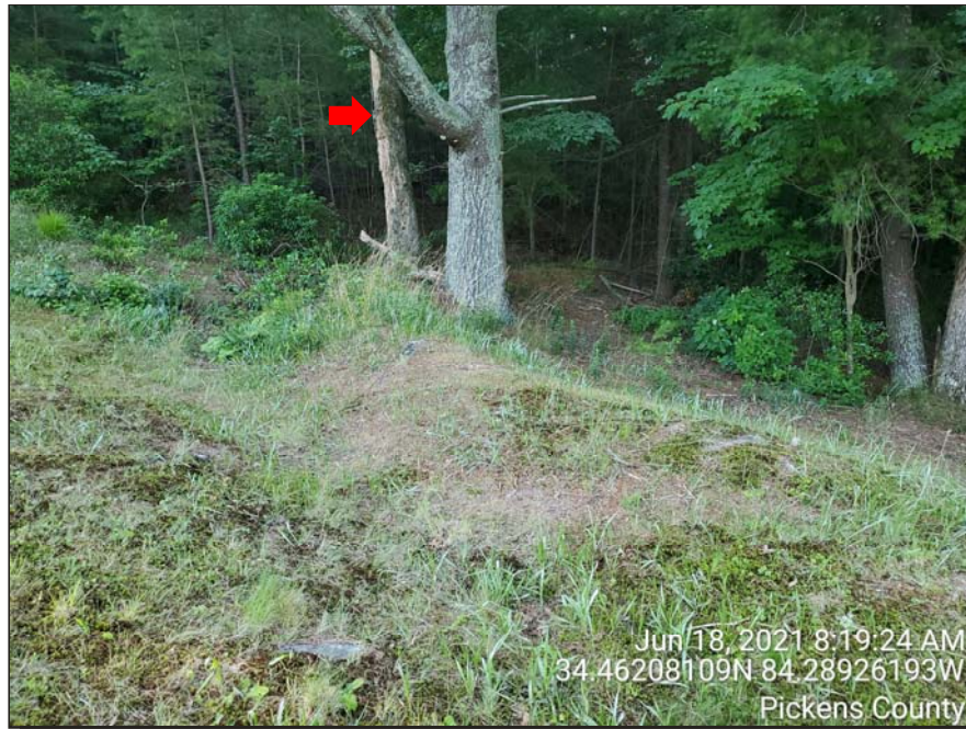
Photograph 7: Downstream face, Jun. 2021 – Surficial erosion with shallow channels developed at Bench No. 4 left abutment. Large dead tree identified during the previous inspection observed in the background.
