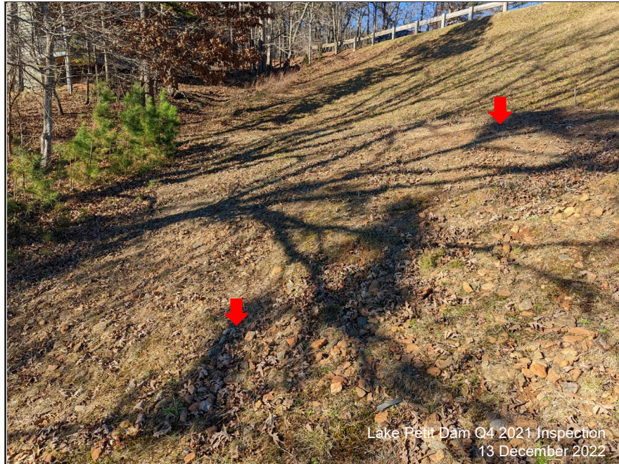
Photograph 3: Downstream Face, Dec. 2021 – Surfacial erosion observed between Bench No.4 and No.5 on the right side of the downstream face.
