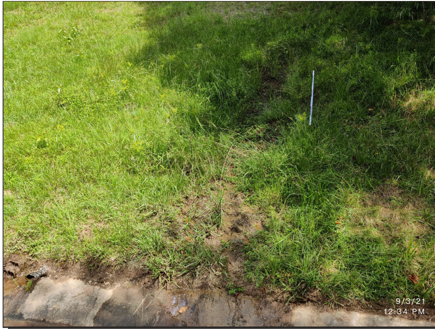
Photograph 5: Downstream face, Sept. 2021 – Previously identified wet area above Bench No. 1 at the left abutment observed to have increased water flow and diminished vegetation from the previous inspection.
