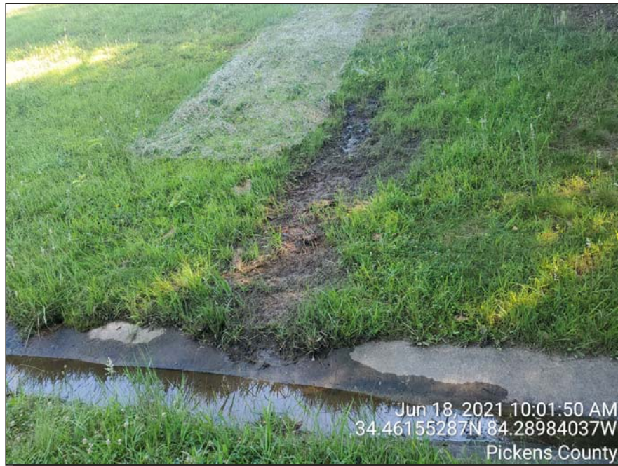
Photograph 5: Downstream face, Jun. 2021 – Previously identified wet area above Bench No. 1 at the left abutment observed to have increased water flow and diminished vegetation from the previous inspection.
