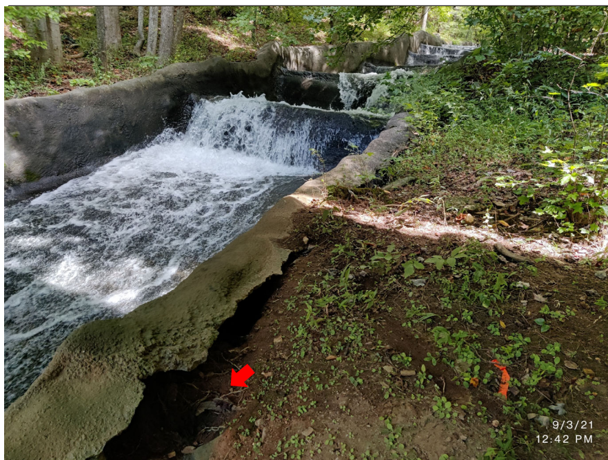
Photograph 4: Spillway, Sept. 2021 – Area of previously identified water flow behind concrete lined channel. Water flow was observed to continue.
