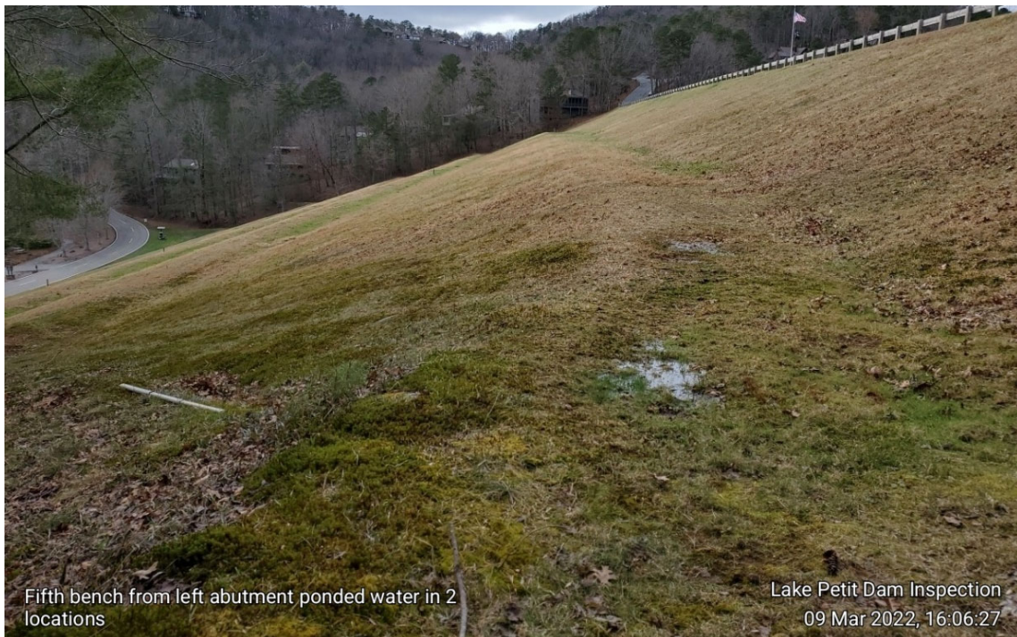
Photograph 23: Bench 5 (El. 1626) minor erosion and ponded water near left abutment
