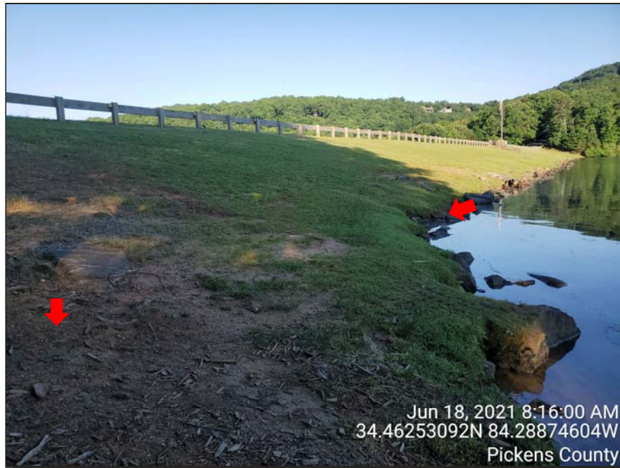
Photograph 1: Upstream Face, Jun. 2021 – localized areas of erosion and beaching along shoreline.
