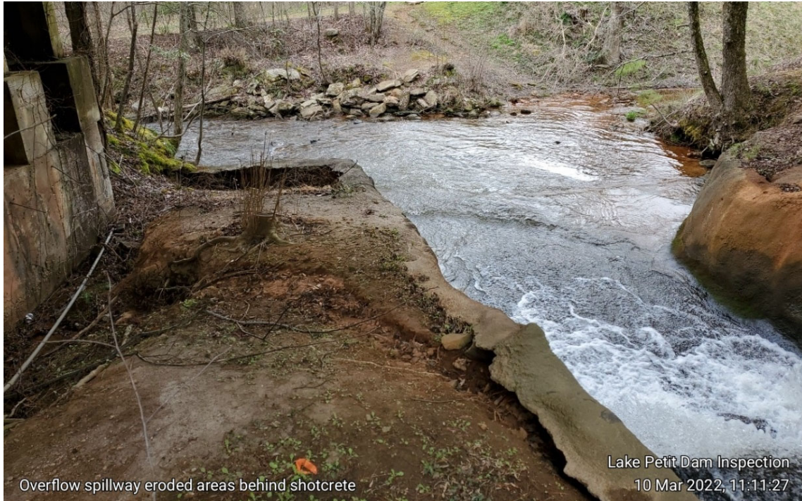
Photograph 29: Eroded areas behind spillway concrete
