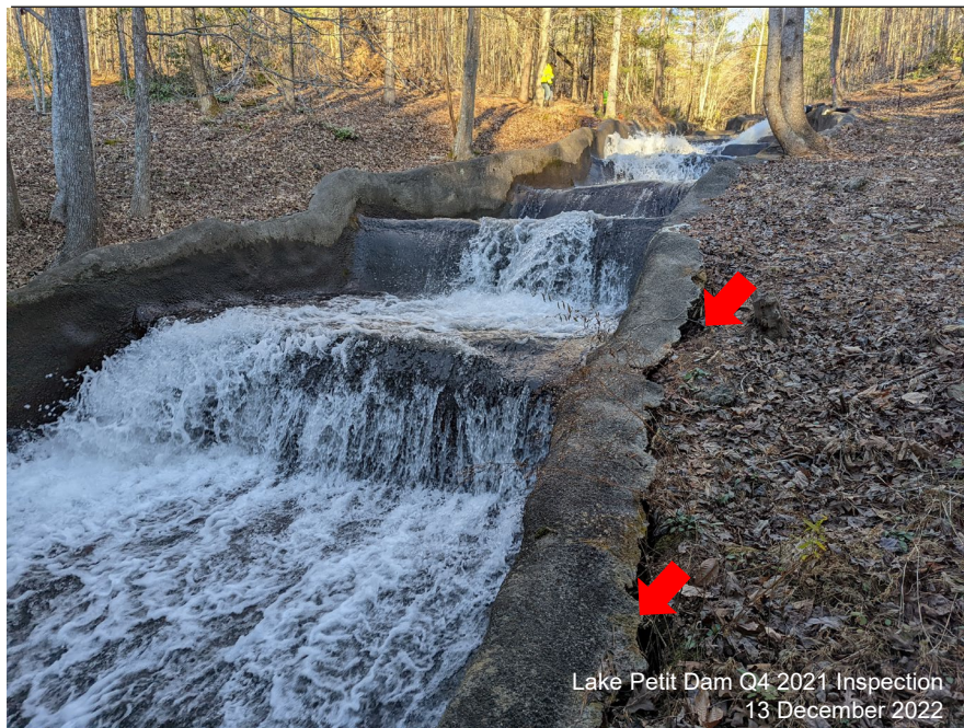
Photograph 8: Spillway, Dec. 2021 – Erosion observed behind the left side of the spillway near the bridge on Wolfscratch Drive. Water was being released via a bypass line operated by Big Canoe to lower the reservoir to conduct a spillway inspection. Maintenance on the spillway is scheduled for early 2022.
