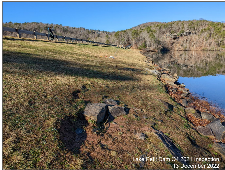
Photograph 2: Upstream Face, Dec. 2021 – Riprap along the bottom of the upstream face is more exposed than previous inspections – shoreline protection repairs are scheduled for early 2022.
