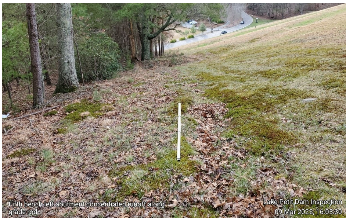
Photograph 22: Bench 5 (El. 1626) minor erosion near left abutment
