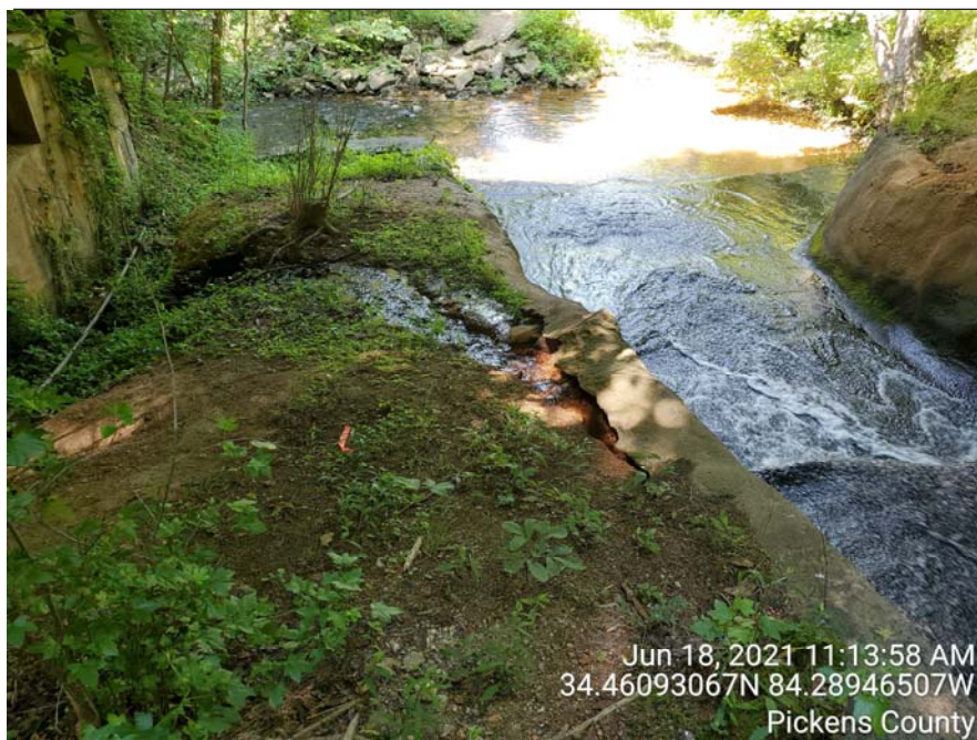
Photograph 4: Spillway, Jun. 2021 – Area of previously identified water flow behind concrete lined channel. Water flow was observed to continue and daylighted at surface in depicted location.
