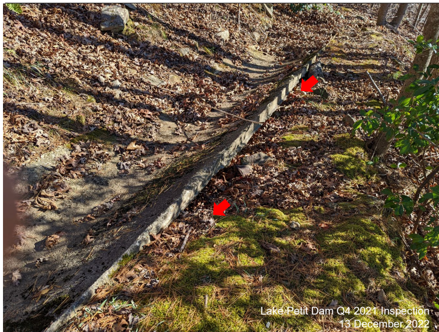
Photograph 4: Left Rim, Dec. 2021 – Foundation material under the concrete channel on Bench No.2 has eroded away, and should be replaced.
