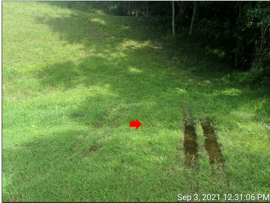
Photograph 7: Downstream toe, Sept. 2021 – Wet area observed at the downstream toe of the dam. The water ponding in the area is believed to be water discharging from the left weir on Bench No. 1.
