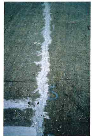
Example of cracking.
