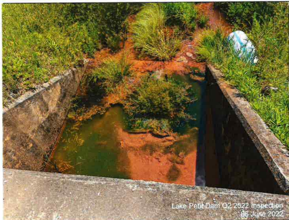
Photograph 4: Impact Stilling Basin, June 2022 – Bacterial growth observed in the instilling basin.
