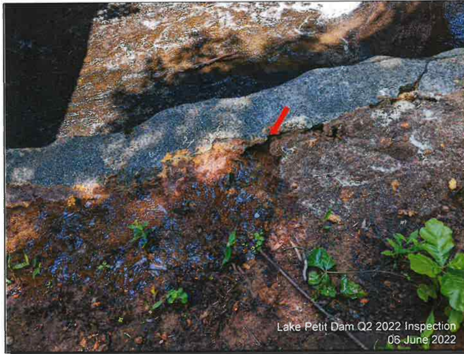
Photograph 5: Spillway, June 2022 – Flow observed on top of the recent repairs conducted in April 2022. The source of the flow is currently being investigated.
