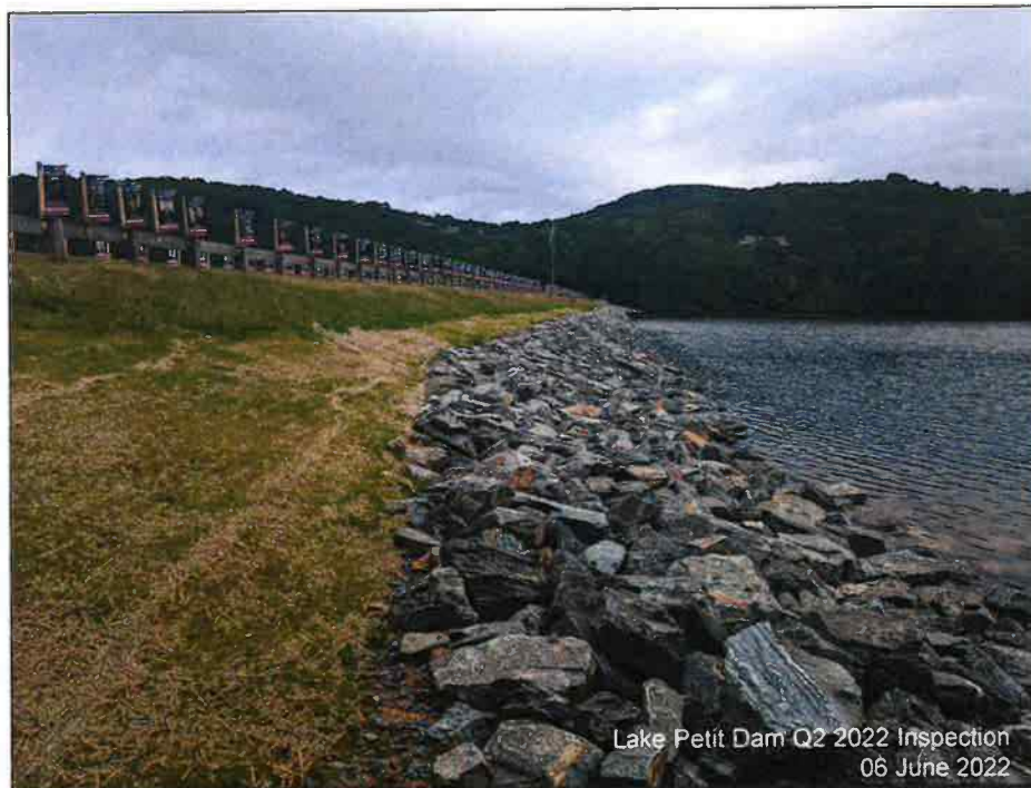
Photograph 2: Upstream Face, June 2022 – Shoreline protection repair conducted in March 2022. No changes were observed on the recently placed rip rap.
