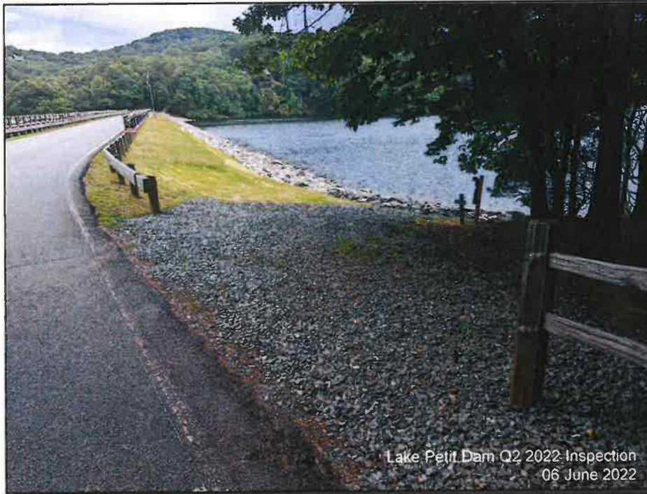
Photograph 1: Upstream Face, June 2022 – GDOT No. 4 aggregate was placed along the left and right groin (not in Photograph 1) to assist with historical surficial erosion observed on the groins.
