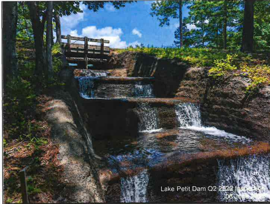
Photograph 3: Overflow Spillway, June 2022 – Flow restored to the spillway after the completion of spillway repairs completed in April 2022. Small leaves were observed in the spillway.
