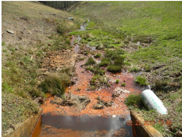
Looking downstream from the low-level outlet with orange ochre in the outlet channel as in past inspections
