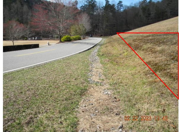
Looking right from near the left abutment at lower downstream slope and toe with saturated area
