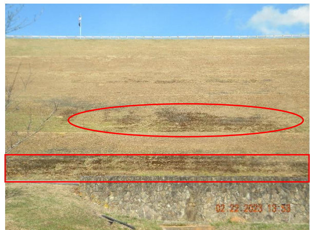
Looking from the right side of the low-level outlet channel at the left downstream slope with saturated areas
