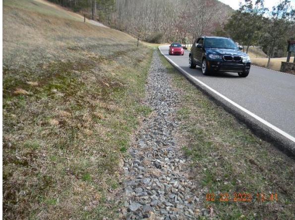
Looking left from near the right abutment at lower downstream slope and toe
