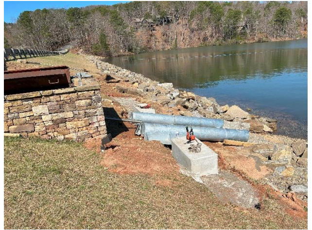
Float and stem below control box.
